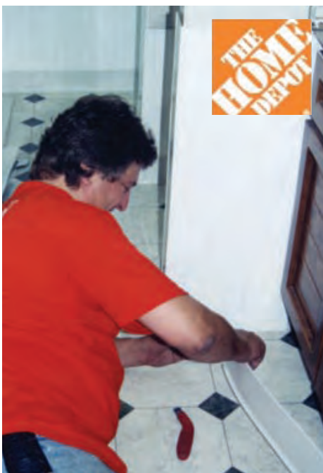
One of a dozen Home Depot volunteers attaches baseboard at the Hartman Home.
